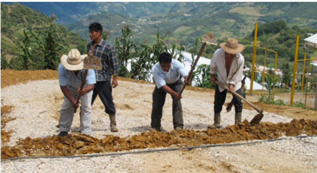
Figure 4.6 The digging of an irrigation ditch at one of the SRC site's affiliated farms
