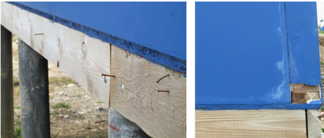
Figure 4.12 The protruding nails and broken exterior walls of an SRC home
