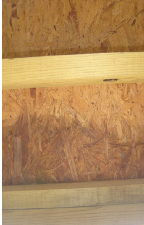
Figure 4.10 OSB floorboard with visible water absorption
