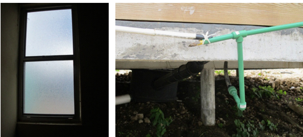
Figure 4.13 The crooked window of an SRC residence (with a visible gap between the window frame and wall)
